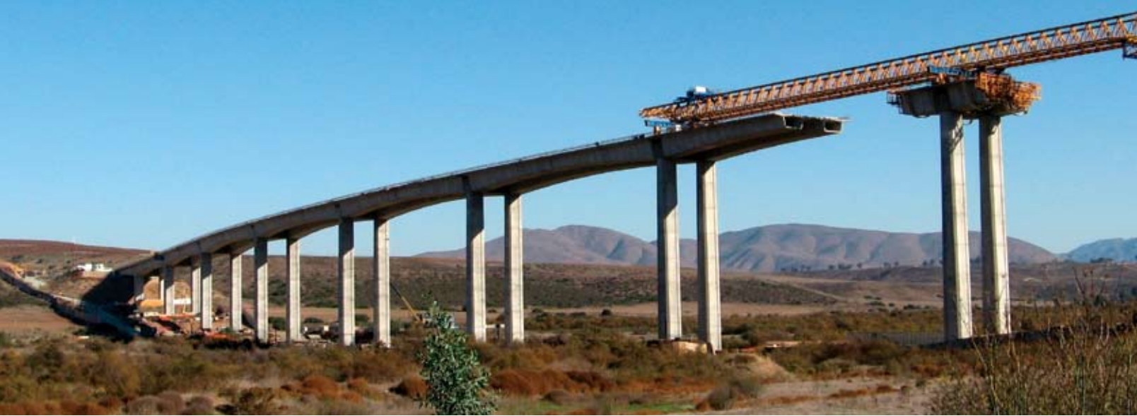
Segments are delivered via an overhead gantry, eliminating the need for falsework.
